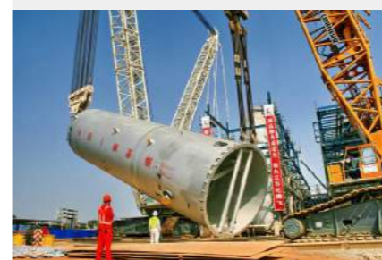
▲ Synchronous lifting and installation of petrochemical pressure vessel in Jiujiang, Jiangxi province.
