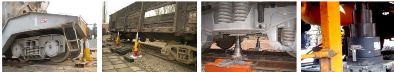
▲ Derailment lifting in position of molten iron transport vehicle in steel plant.
