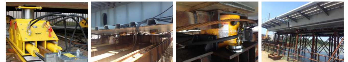
▲ Synchronous pushing of large steel box culvert structure in high speed rail construction. ▲ Synchronous pushing and installation of steel box girder in bridge construction. ▲ Synchronous pushing and installation of steel box girder in bridge construction. ▲ Synchronous pushing and installation of steel box girder in bridge construction.
