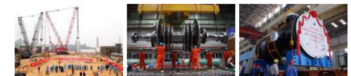
▲ Hoisting of pressure vessel in oil refinery. ▲ Hoisting of steam turbine in thermal power plant. ▲ Hoisting of nuclear power equipment.
