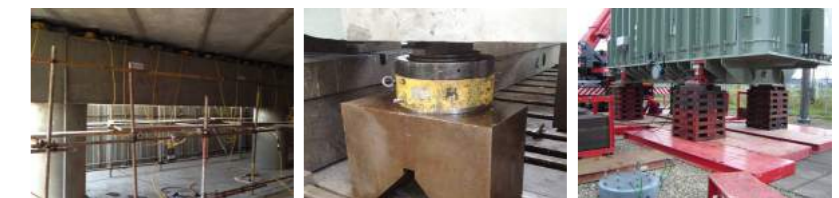
▲ Bridge repairing and replacement of rubber bearings. ▲ Long time support for large equipment maintenance. ▲ Long-term lifting support for large transformer.
