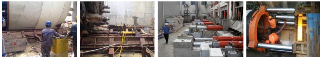
▲ Synchronous pushing of shield machine. ▲ Synchronous pushing of shield machine. ▲ Synchronous pushing and translation of historic building. ▲ Trenchless underground pipe pushing.
