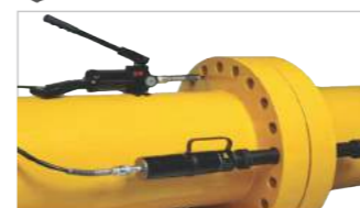
▲ Pipeline flange separation in refinery.
